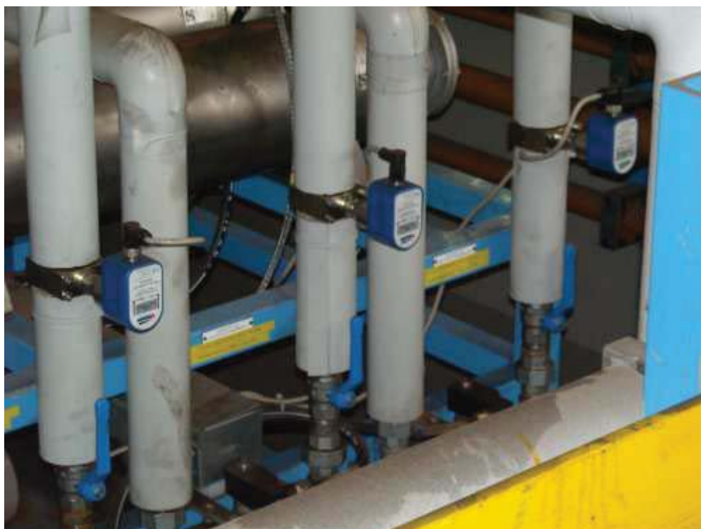
Picture 4: Control of a lubrication oil line with flow rate sensors fluid-Check ® and serv-Clip ® -2 at a continuous pickling line.
